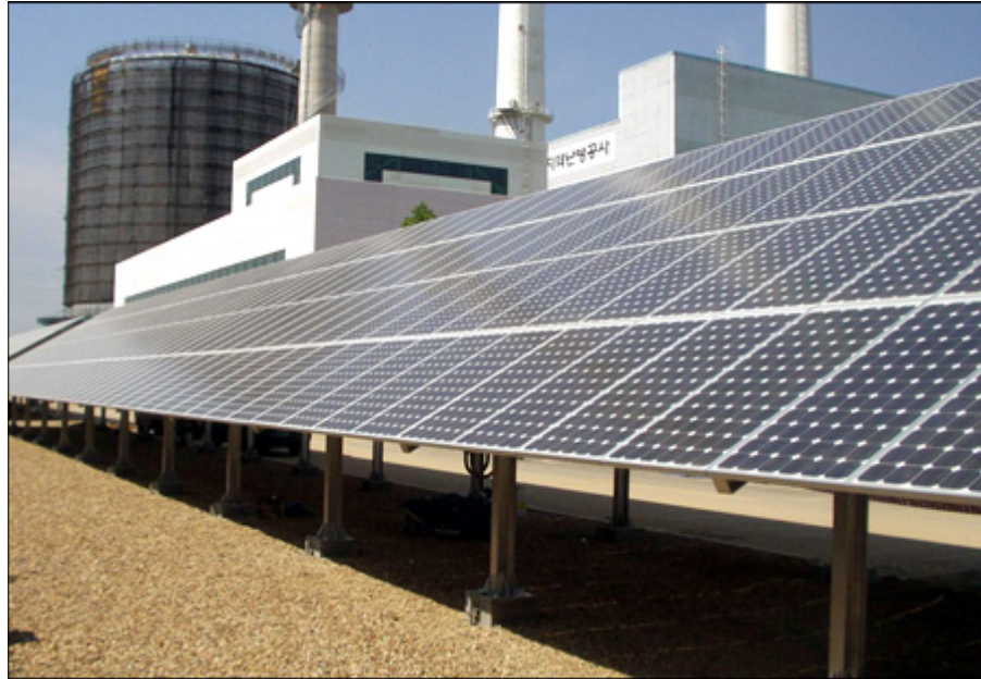
Solar panes are designated as one of top priorities under Korea's alternative energy plan. / Korea Times
