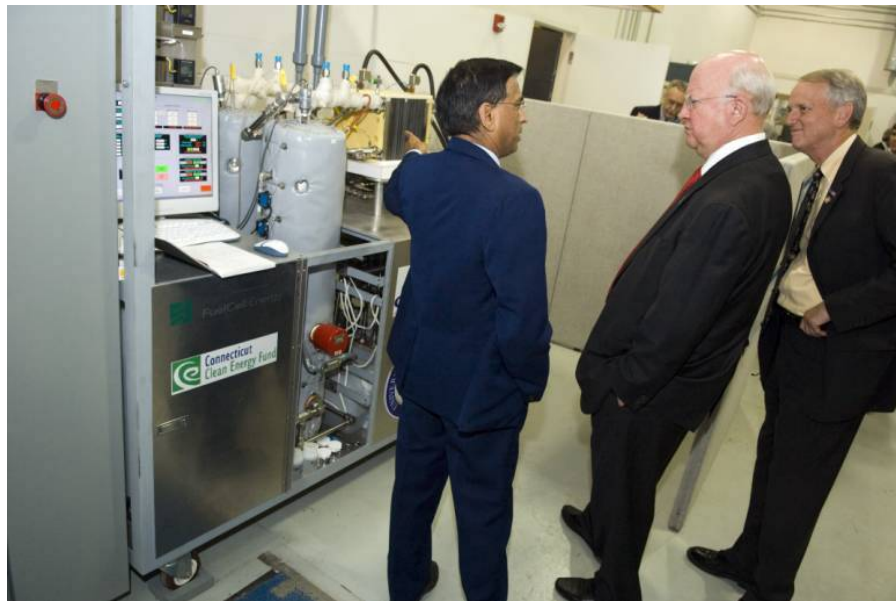
Figure 2. FCE's EHS System in Operation at the University of Connecticut: P. Patel of FCE (left) demonstrates elements of the EHS System, producing 30,000 liters/day of hydrogen, to U.S. Energy Secretary Samuel W. Bodman (middle) and U.S. Rep. Rob Simmons (R-Conn.)
