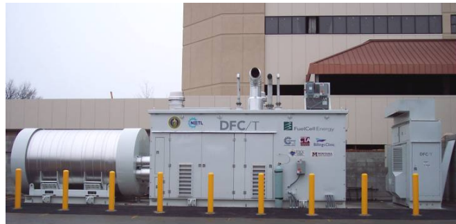
Figure 2. Alpha DFC/T Unit Installed at the Billings Clinic, Montana Demonstration Site
