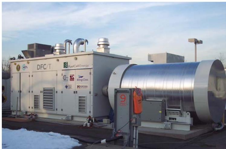
Figure 5. The First DFC/T ® Power Plant during Factory Alpha Testing
