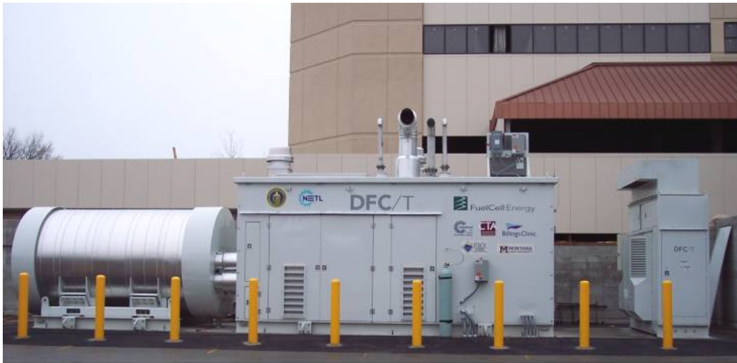
Figure 4. Alpha DFC/T Unit after Installation at Billings Clinic, the Montana Demonstration Site
