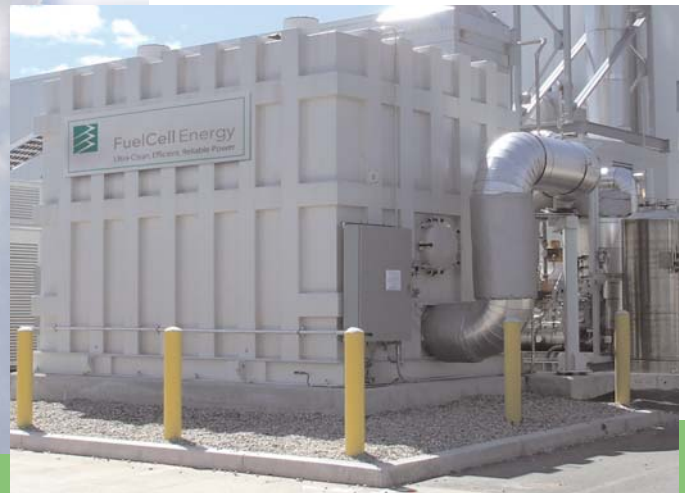
1.4 MW DFC Power Plant at Pepperidge Farm Bakery in Bloomfield, Connecticut
